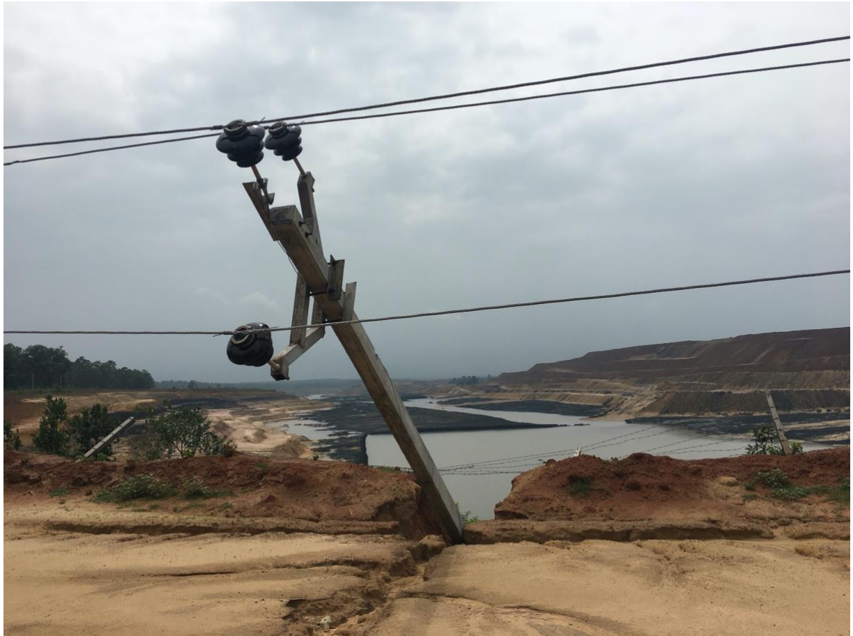
Figure 14: Broken electricity pole against a coal mine in Chhattisgarh
