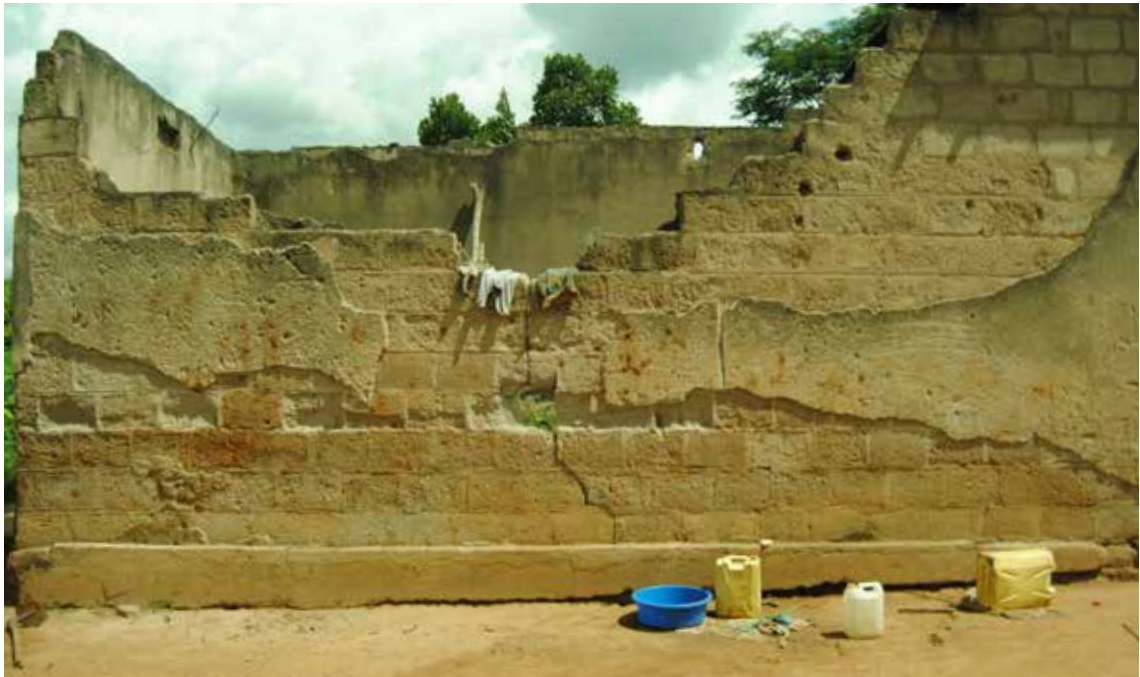
Figure 1.3 Bombed co-operative store house. The roofing raided by NRA to make shelters.
