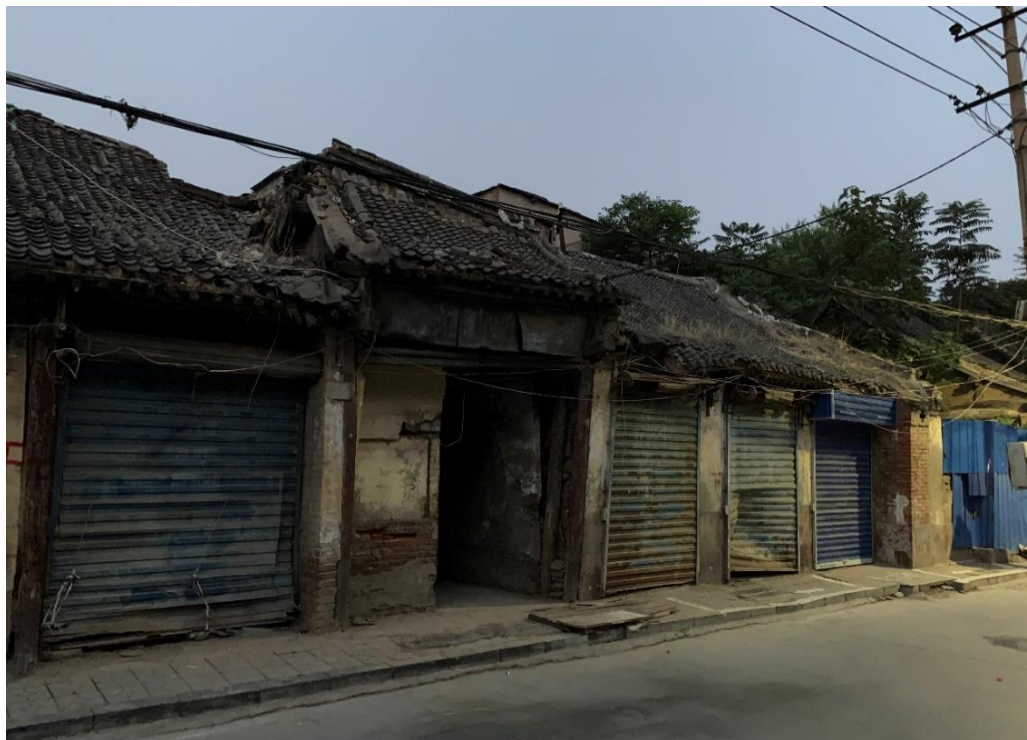
Figure 5-2. Empty and dilapidated buildings on South Street (Source: author, 2021).
